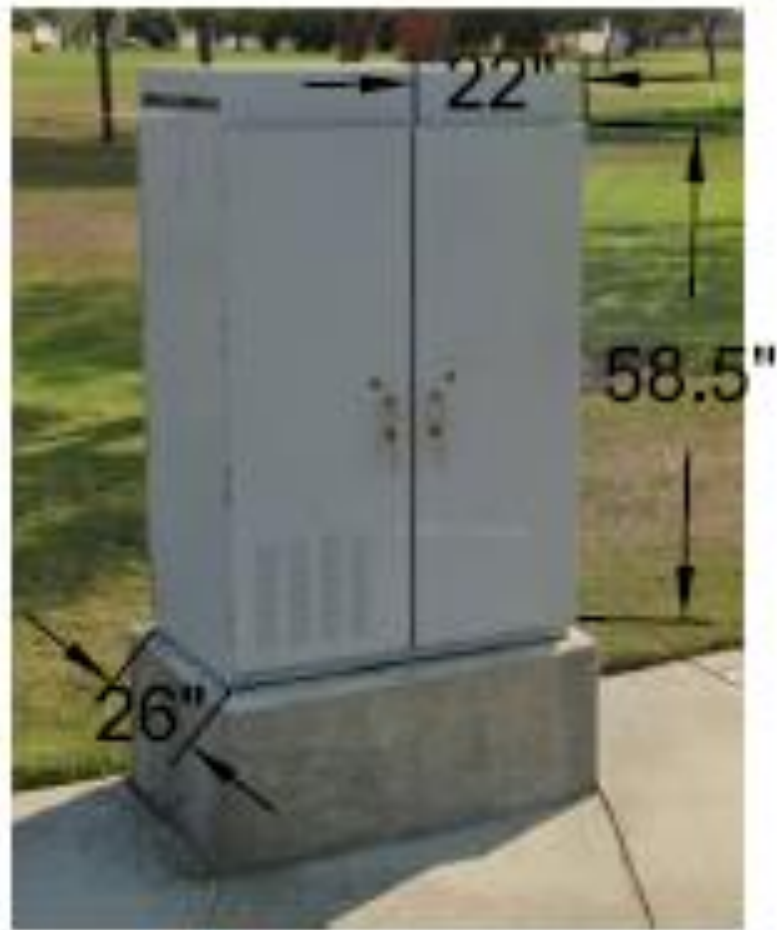
● Type 333 Traffic Signal Cabinet (39)
